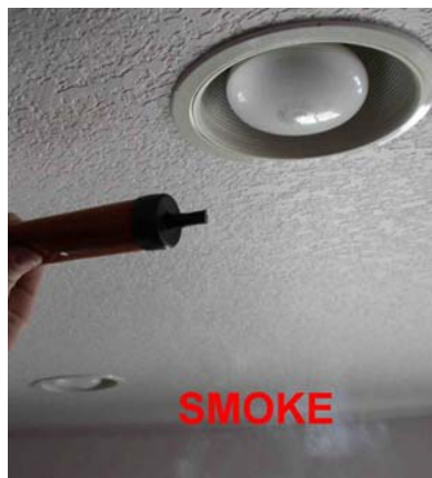
Figure 4. Can light in a kitchen ceiling with a blower door depressurizing the home. Smoke indicates openings to the vented attic above.
