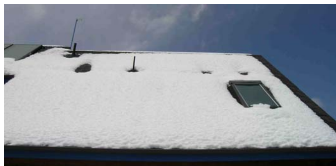
Figure 7. The two holes in the snow above the skylight correspond to recessed can lights in a bedroom that are almost never turned on. Melting is due only to air exfiltration from the conditioned space below the cans and the lack of insulation on top of them. The larger melted hole in the snow to the left of the vent pipe is due to a similar can above the shower which has a 250 watt infrared bulb in it. This light is on a timer and on average is illuminated about 12 minutes a day.
