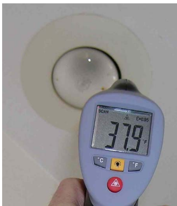
Figure 6. Kitchen light in a home heated to 68°F, outside air temperature of 34°F, blower door depressurizing the home
