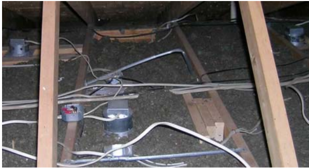
Figure 15. Leaky cans crisscrossing poorly-insulated attic
