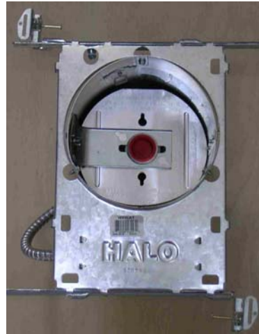
Figure 16. Example of new IC can installed. This air tight can costs only a dollar or two more than those that are unsealed.
