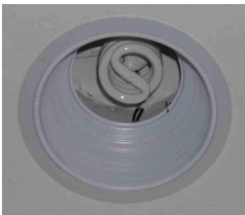
Figure 13. White painted reflector with 23 watt spiral CFL
